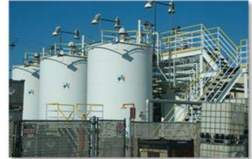
Outside Tank Farm Bulk Storage
